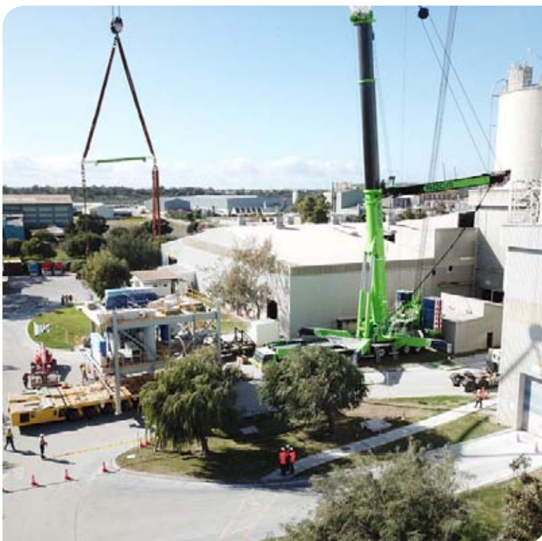
Below: Cockburn Cement and HAVER & BOECKER took an innovative approach to the installation of the Kwinana plant’s new bagging and palletising line.
